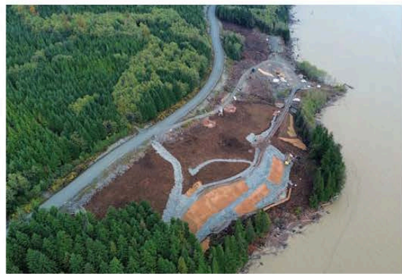
Aerial view of the marine terminal area showing clearing work and environmental measures completed prior to construction in 2025.
